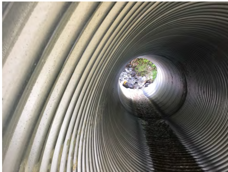
Culvert slightly misaligned at coupled location
